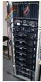
amp rack with ALC2' s
